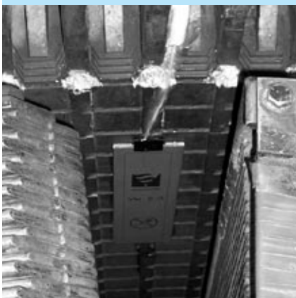
2005 – VM 5.0 air gap sensor seen between two rotor poles of a hydrogenerator.
