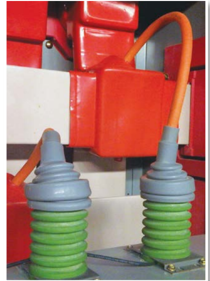
Installed Capacitive Couplers
