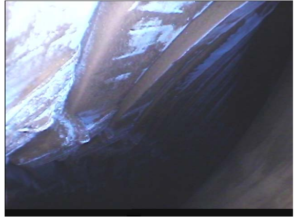
Figure 16: Drive End - Lower Endwinding with Dirt and Oil
