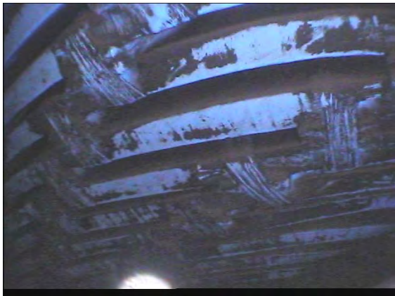
Figure 14: Drive End - Lower Endwinding with Dirt and Oil
