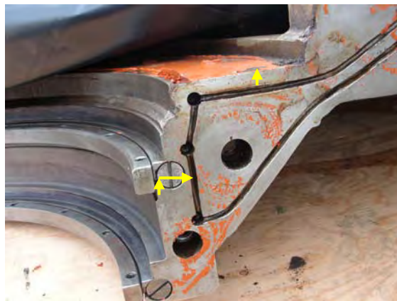
Figure 10: Upper Endshield Horizontal Flange - Arrow Shows Oil Path to Generator from Bearing Seal Cavity
