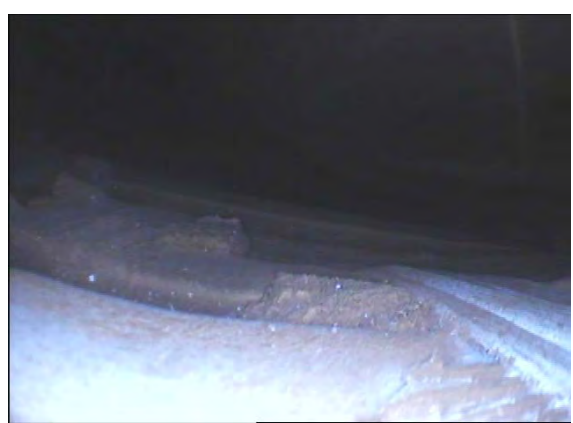
Figure 18: Non Drive End - Lower Endwinding with Dirt and Oil
