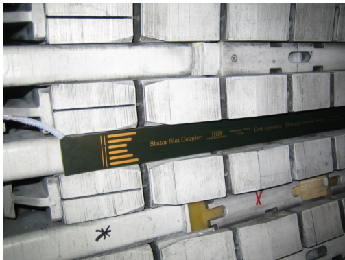
Fig 2: An SSC antenna in the process of being installed on a large generator. A stator wedge is inserted over the antenna.
