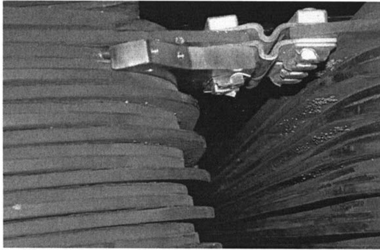
Example of a temporary shorted turn placed on one pole of a 330 MW machine with a strip on edge winding.
