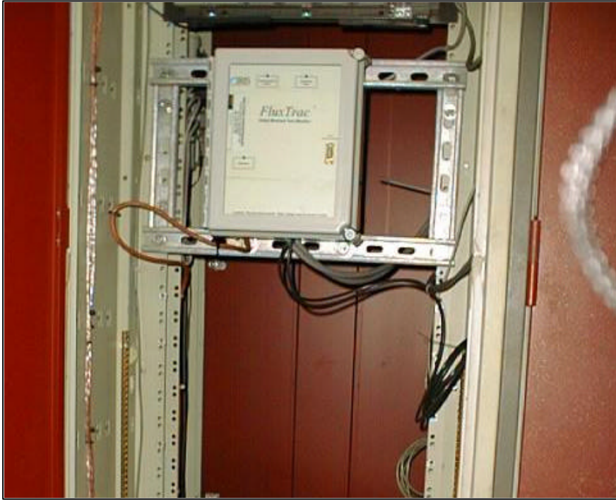
Figure 1: FluxTrac installed at convenient location in plant
