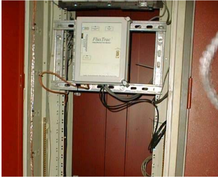
Figure 5: Continuous flux monitor installed centrally to generators to be monitored.
