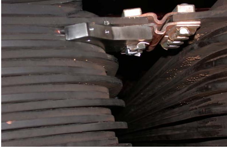
Figure 2: Example of a temporary shorted turn placed on one pole of a 330 MW machine with a strip on edge winding.
