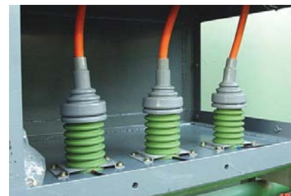
Installed Capacitive Couplers
