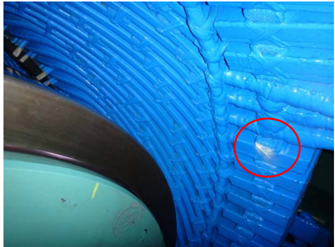
Figure 1 – Dusting Between Felt Block and Stator End Cap
