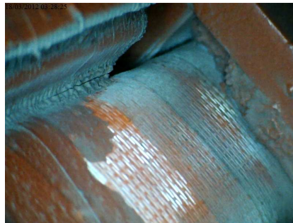
Figure 8. Surface PD Activity – Voltage Stress Coating Deterioration
