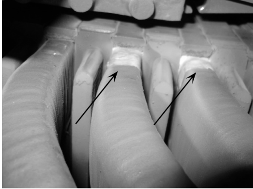
Figure 7. Damage to Voltage Stress Coating
