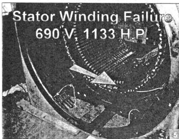
Picture of Motor 1 after failure.
